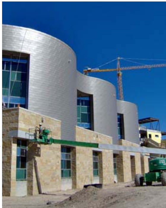
Metal panels and limestone sheathe the exterior of the inpatient room wings. The curved shape will enable views of the outdoor healing garden. (Photo courtesy White Construction.)
