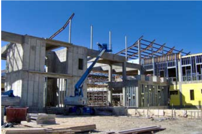
Crews work on the final touches of the structural concrete shell of the Dell Children's Medical Center and begin adding exterior finishes. (Photo courtesy White Construction.)
